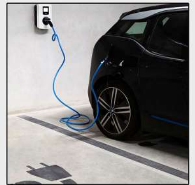
EV Charging Points
